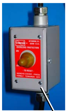
Remote Power Switch (Variable Speed Controller Optional)
